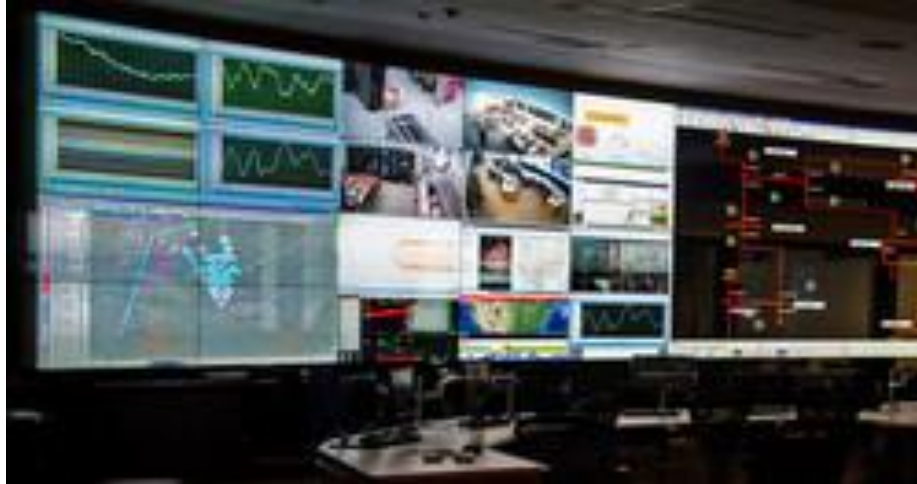
Figure 5. PNNL's Electricity Infrastructure Operations Center
