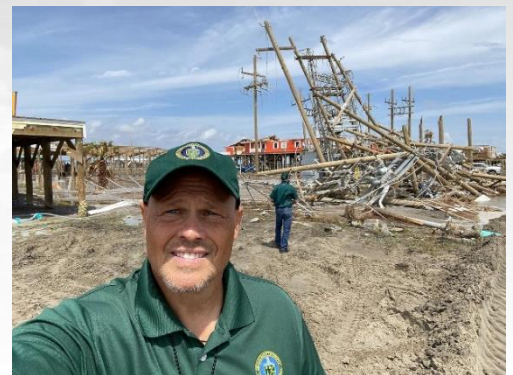
ESF#12 responder Russ Haffner assessed damage in Louisiana after Hurricane Ida.
