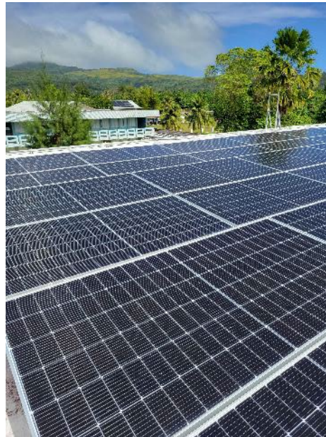
Figure 11. Solar PV Installed at a Marianas High School Building
