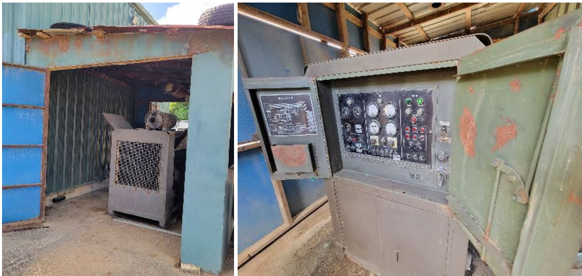
Figure 43. Rental Generator in Enclosure with Some Corrosion
