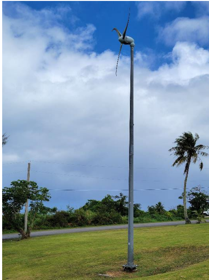
Figure 18. Skystream 2.4 kW Wind Turbine at DPW Building
