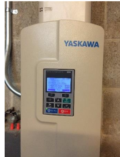
Figure 6109PAS.3 Garage Fan VFD
