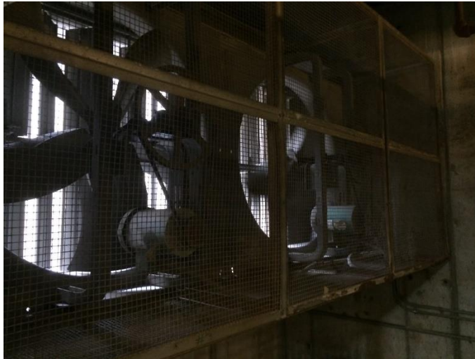
Figure 6109PAS.2 Garage Exhaust Fans
