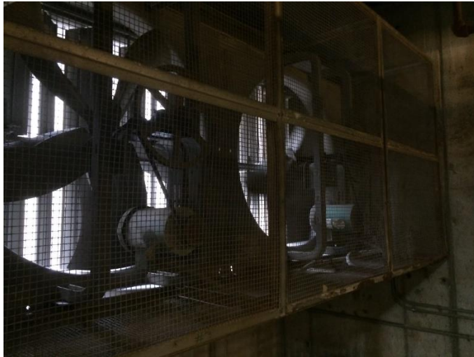
Figure 6109PAS.2 Garage Exhaust Fans
