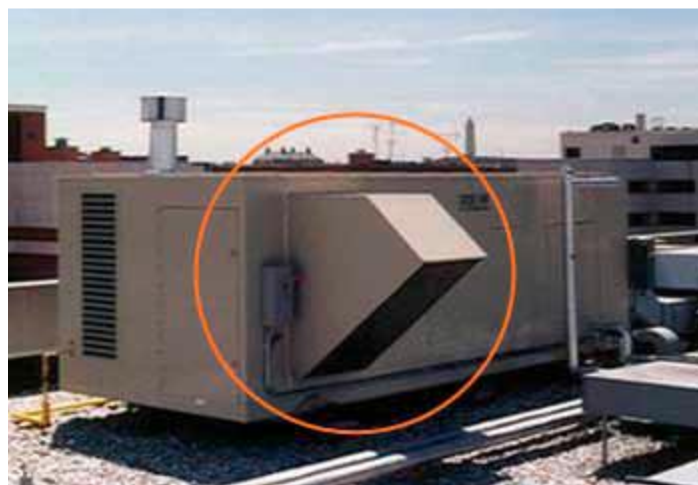
Figure 6066P.1 Outside Air Ductwork for Air Economizer 1
