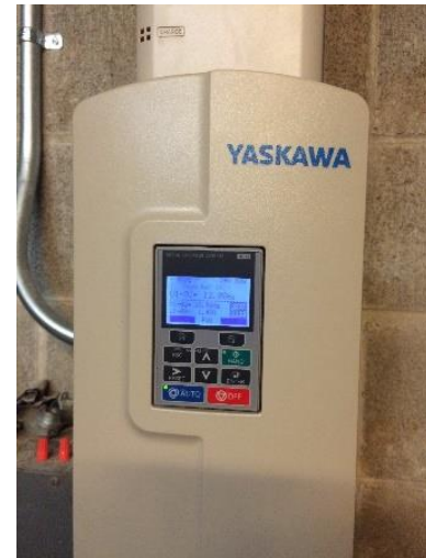
Figure 6109PAS.3 Garage Fan VFD
