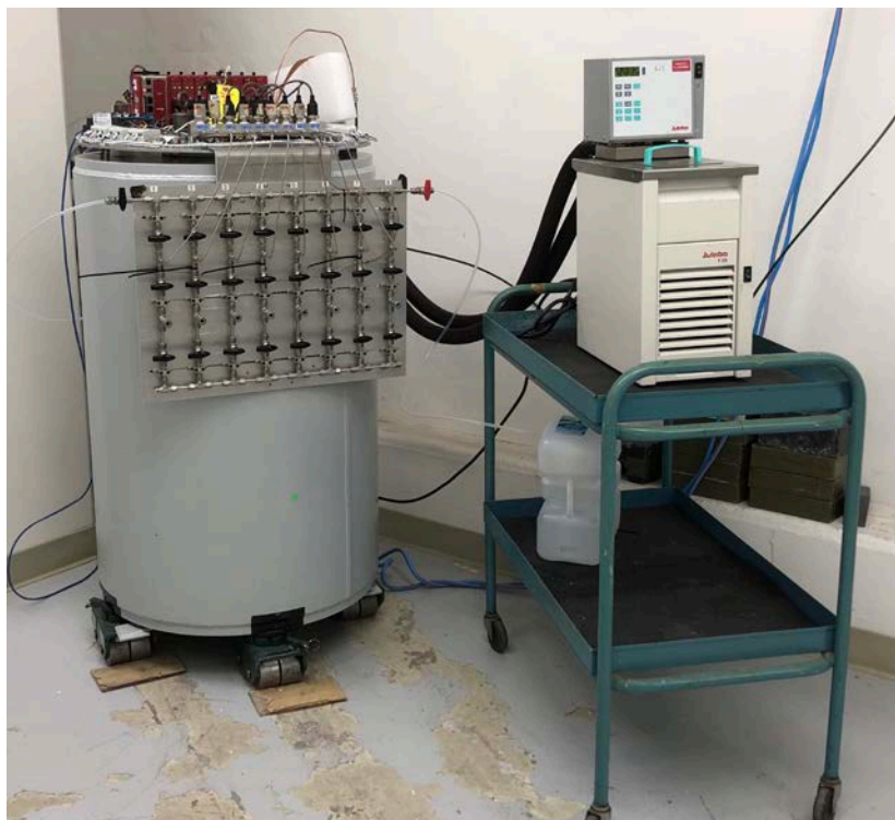
Figure 4.1. Rad system bunker with the updated chiller installed
